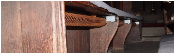
Chancel choirstalls: three 320 W ARCAngel SOLACE units beneath each stall.
