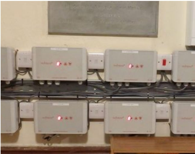
The nine installed regulators on the west nave wall. A cabinet to conceal the units and wiring, and to prevent casual misuse, remains to be built. See lesson 05.
