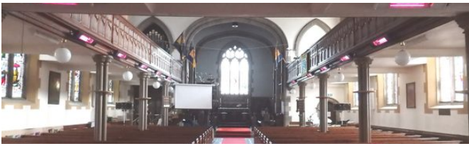
In service, looking east. Black units on the gallery fronts, white units on the beams beneath.
